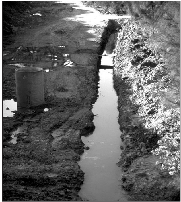
Construction of a leachate drain for waste at Homebush Bay. (photo by Sharon Beder)
